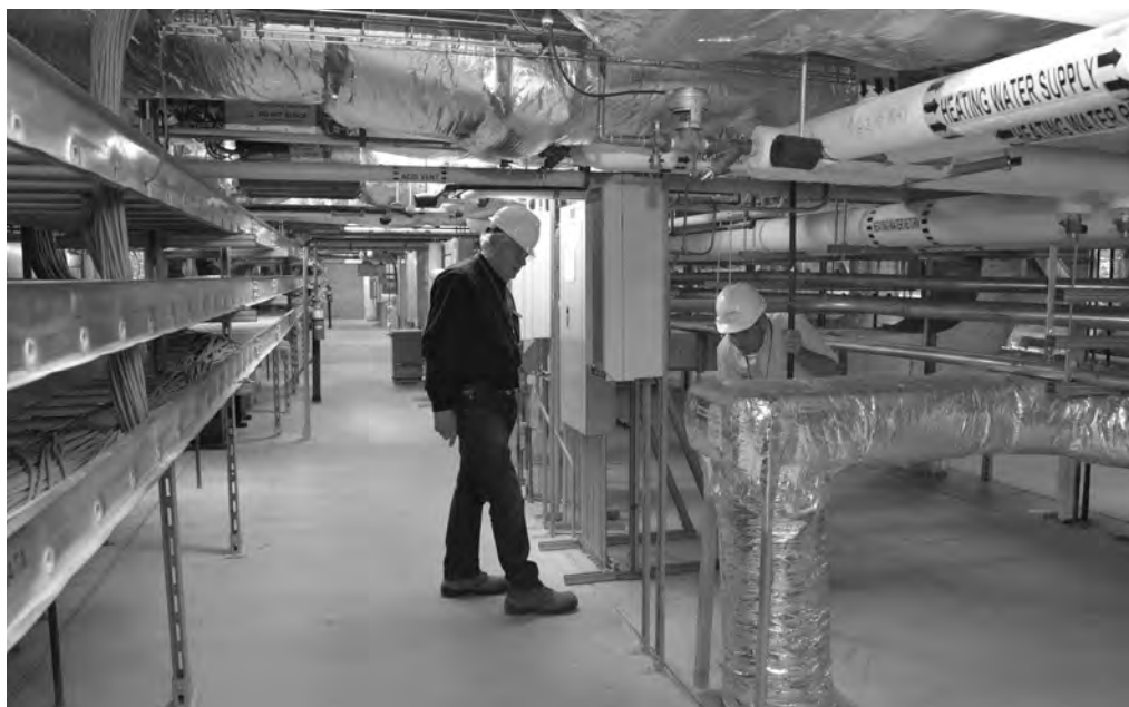
Jim Wilson (left) and Fred Manuel visit the Hatfield Building's dedicated mechanical space on the second floor to check on an exhaust pipe that manages air flow in the laboratory below.
